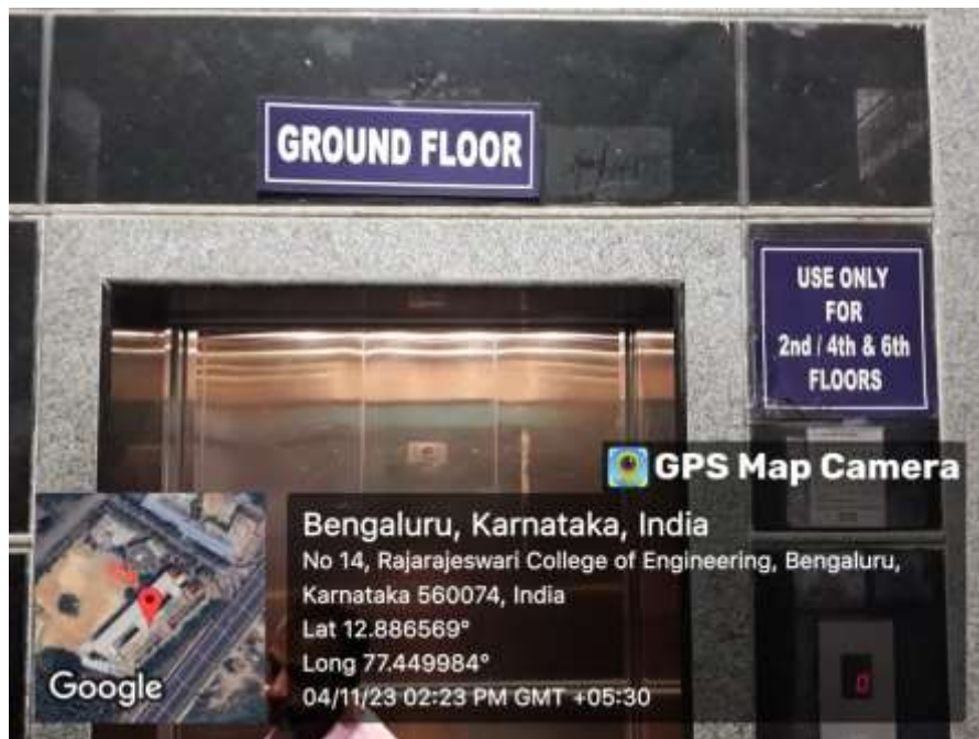
Photo.2: Lift facility inside the college
