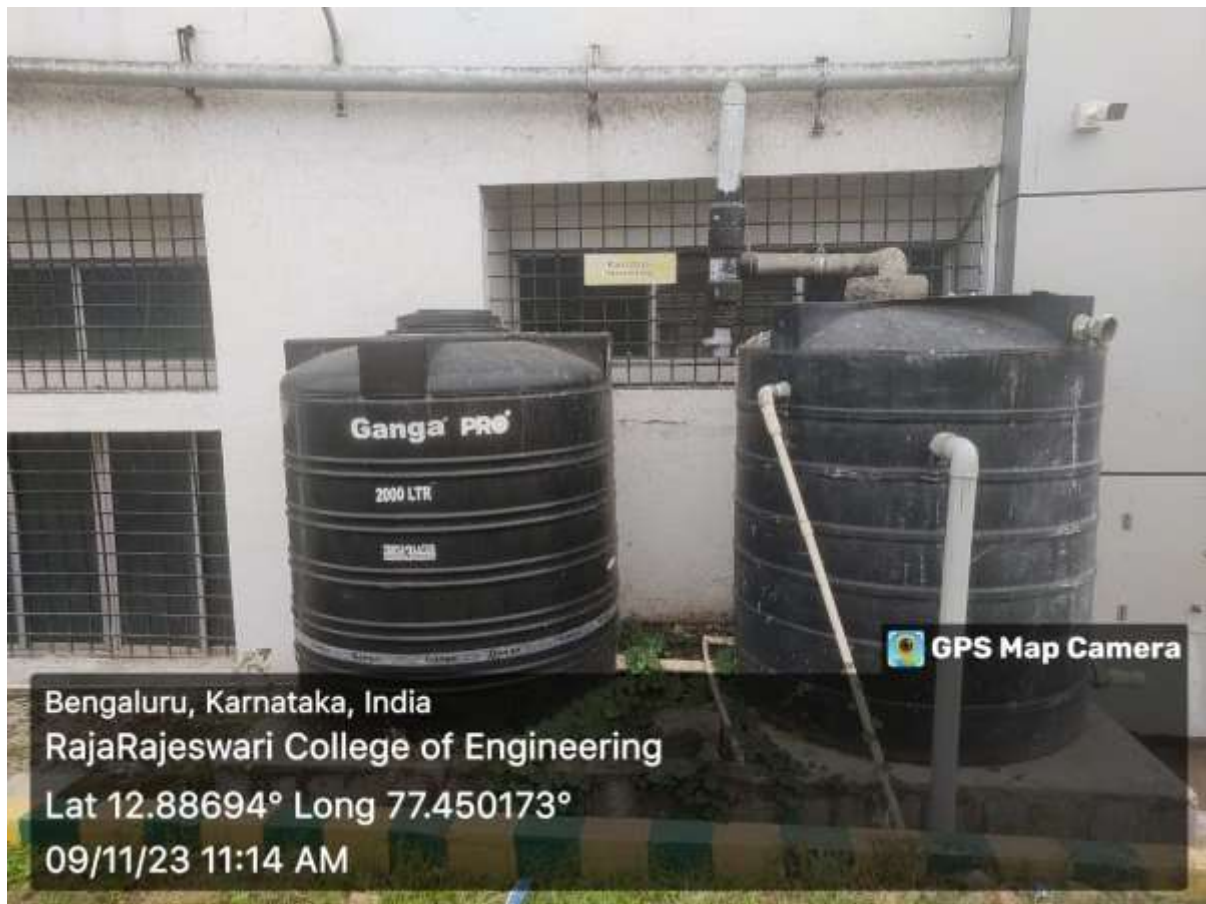
Photo.1: Rain water harvesting facility inside the campus
