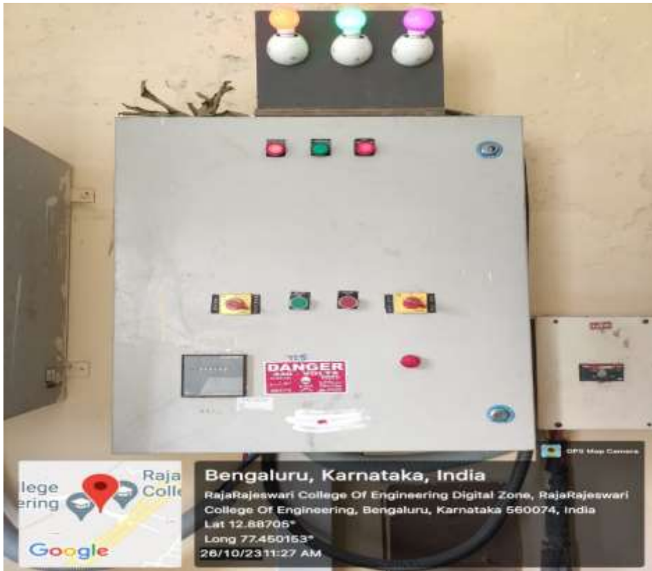
Photo.4: Sensor based water pump systems in Rajarajeswari College of Engineering
