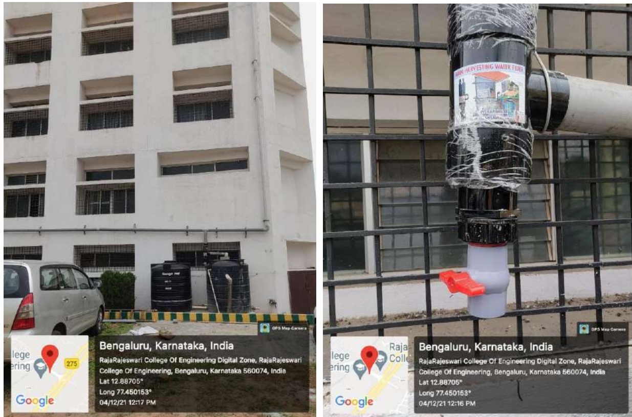
Photo.2: Rain water storage tanks and rain harvesting water filter
