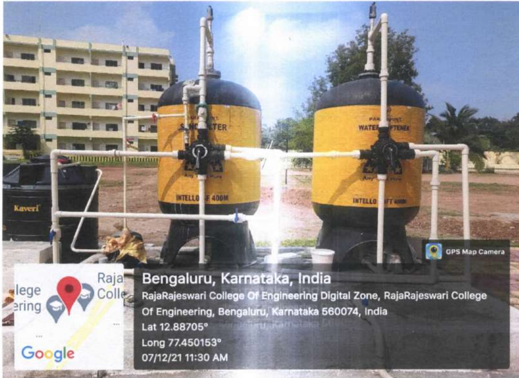
Photo.5: Water filter and Water softener plant installed in the campus
